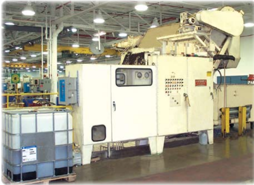
Mixing station that serves Vought's 13,000 gallon flume
